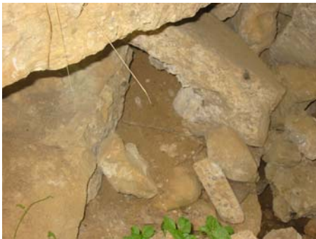
Raveling into open voids.
