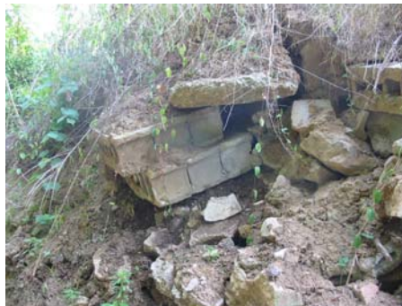
Collapse & poor compaction.
